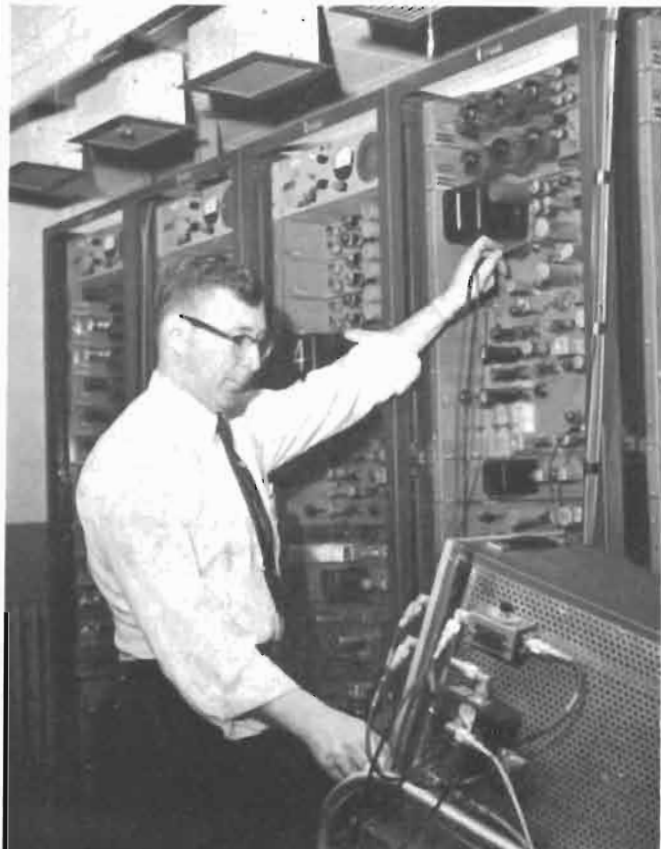
The awesome array of electronics required for proper color operations requires steady maintenance using the very latest in test equipment. Here a technician adjusts a colorplexer.
